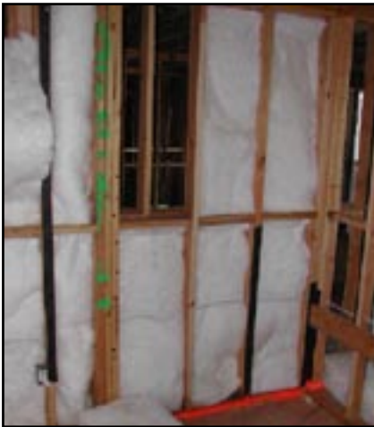
Materials: Batt insulation
